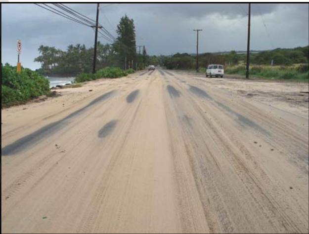
Evidence of waves overtopping Kamehameha Highway at Laniākea Beach (January 29, 2007)
