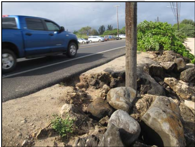
Coastal erosion at Laniākea Beach
